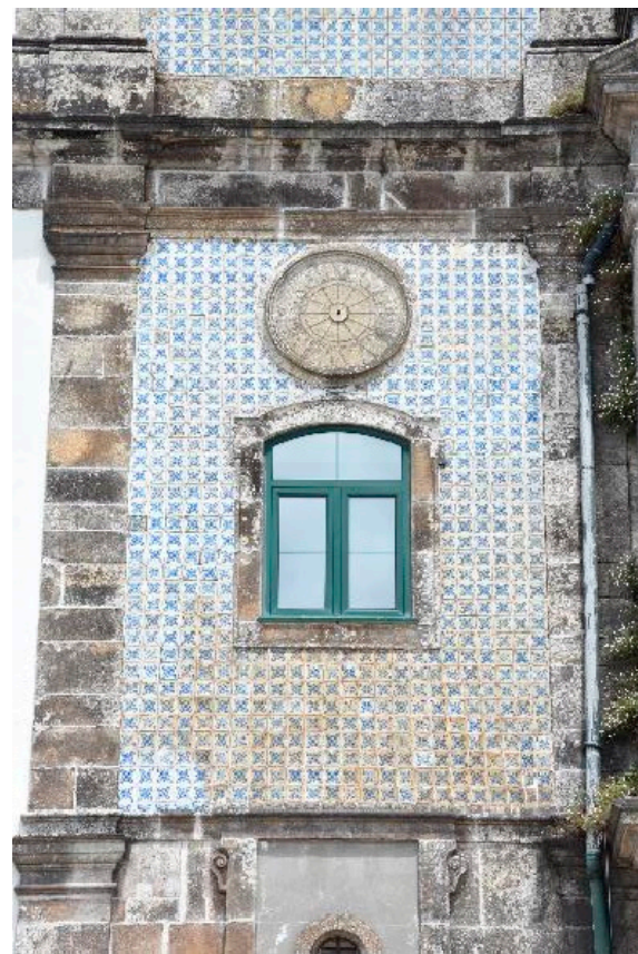
Figure 16. Details of the anomalies present on the south facade of Carmelitas Church. Source: author.
