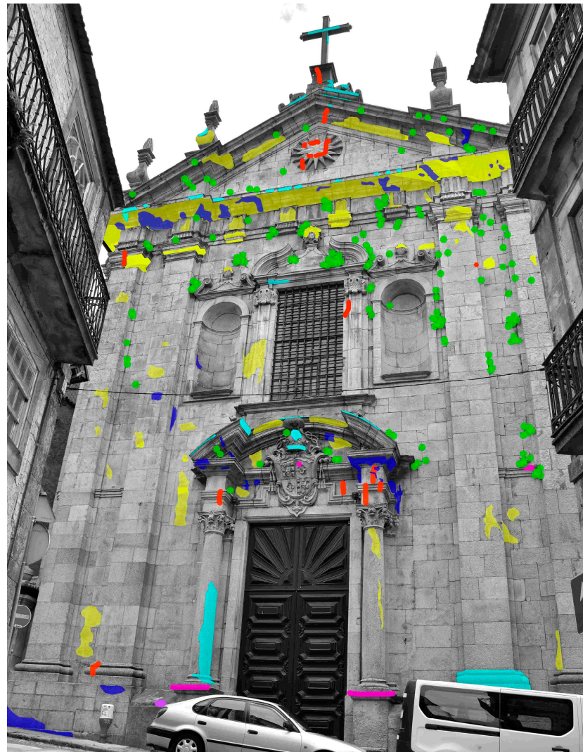
Figure 31. Anomalies map on the front facade of Vitória Church. Source: Author.
