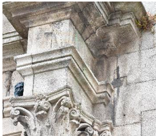
Figure 28. Identification of the various pathologies on the north façade of Vitória Church, Porto. Source: Author.
