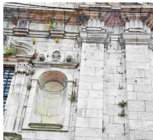
Figure 29. Identification of the various pathologies on the north façade of Vitória Church, Porto. Source: Author.
