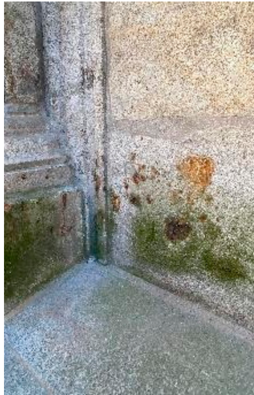
Figure 22. Identification of the various pathologies on the north facade of São João Novo Church. Source: Author.
