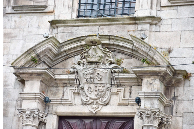
Figure 27. Identification of the various pathologies on the north façade of Vitória Church, Porto. Source: Author.
