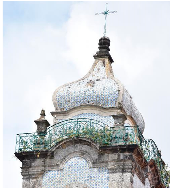
Figure 15. Details of the anomalies present on the south facade of Carmelitas Church. Source: author.
