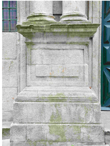
Figure 20. Identification of the various pathologies on the north facade of São João Novo Church. Source: Author.
