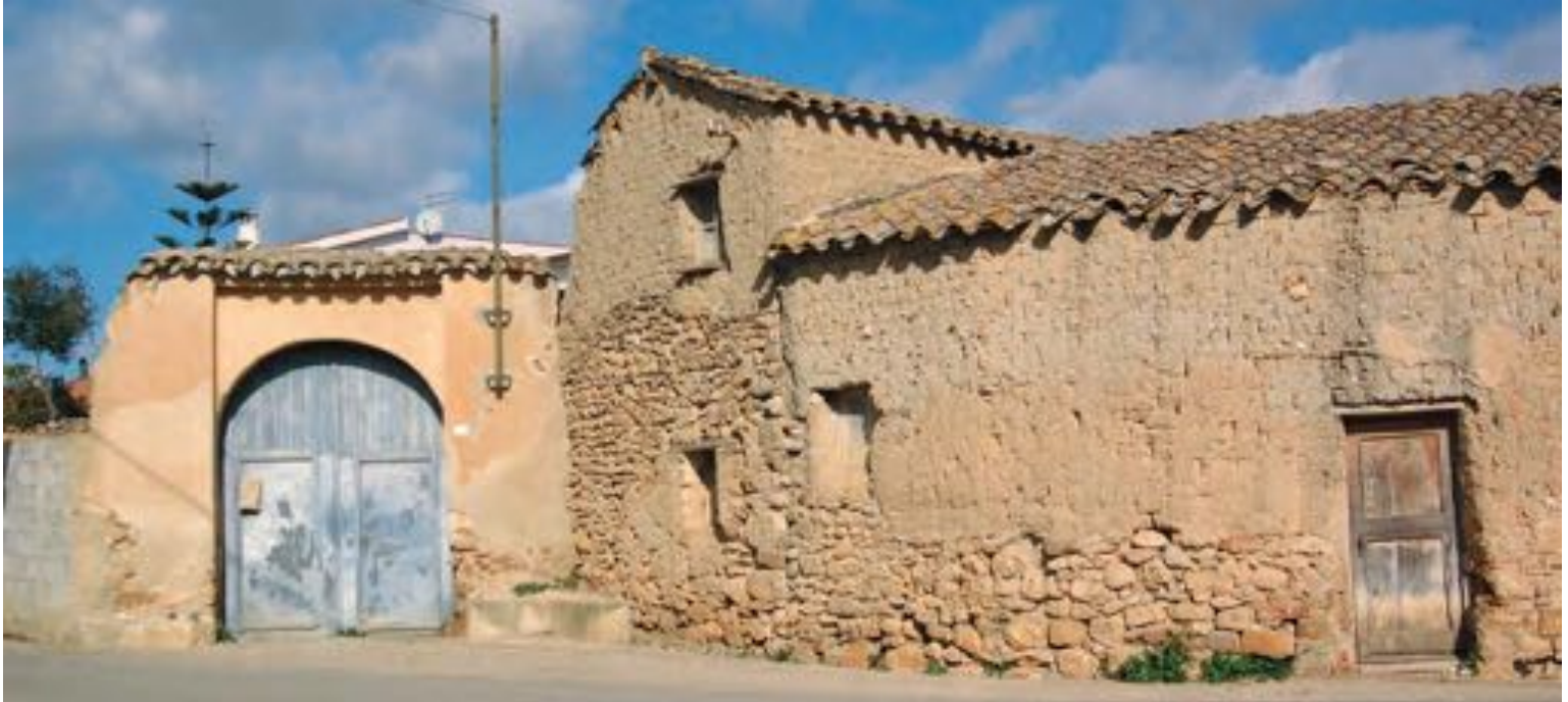
Traditional house in adobe (domu) in Samatzai, Sardinia, Italy. (photo: Silvia Onnis) Adobe houses in Sambiasse, Calabria. (photo: Ettore Pelaia)
