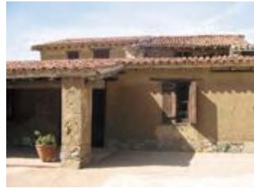
Traditional adobe structure restored by the Cyprus Department of Antiquities, Fikardou Cyprus. This restoration project has received a Europa Nostra Award
