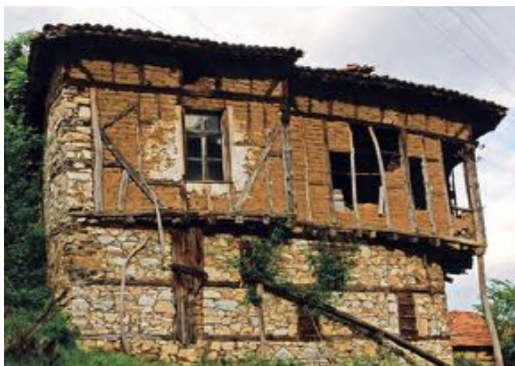
Houses built with stone, adobe and wooden beams in the region of Gotse Delchev. (photos: Saverio Mecca)
