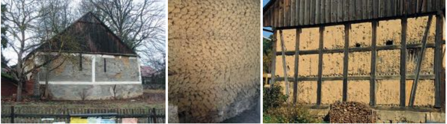
Examples of historical building techniques: adobe masonry, clay rolls opus spicatum, half-timbered structures with wattle and clay. (photos: Žabičková Ivana, Růžička Jan)
