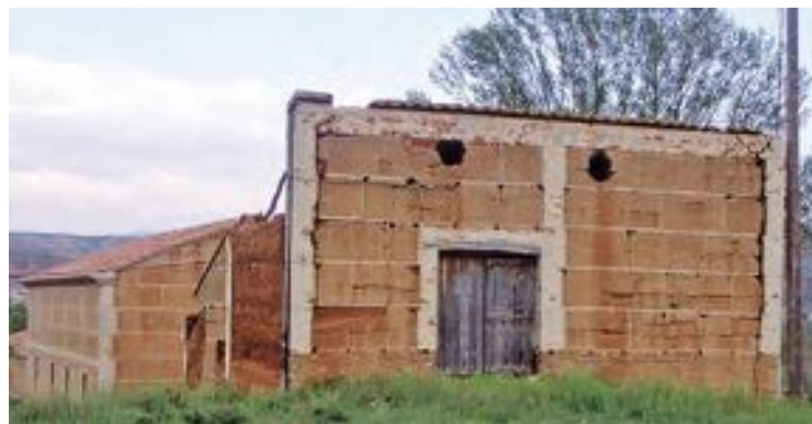
Example of rammed earth wall in rural house, Jijoca, Teruel, Aragón. A dovecote ( palomar ) in Tierra de Campos (Castilla y León). (photos: Juana Font)
