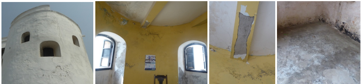
Figs. 177 to 180 – Concrete beams were inserted in the entrance tower which are not strong enough to hold the concrete 2 nd floor.
