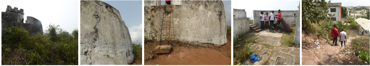
Figs. 143 to 147 – Fort Victoria is surrounded by bushes (fig.143), has some structural cracks (fig.144), foundations exposed and fragile metal stairs (fig.145), vegetation growing inside the fort (fig.146) and an unclear access to the fort (fig.147).
