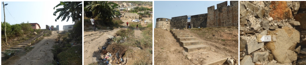
Figs. 97 & 100 – Access to Fort Amsterdam in Abandze (figs.97, 98 & 99), and a crack monitor device to measure fissures (fig.100).
