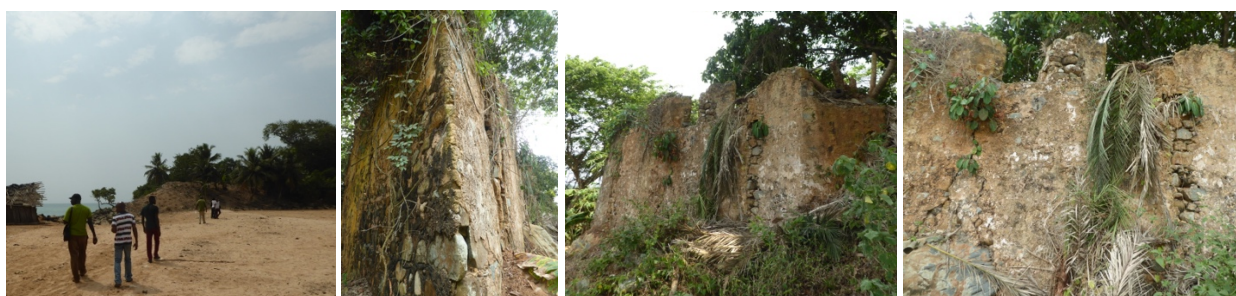
Figs. 202 to 205 – Access to Fort Dorothea (fig. 202); and structural problems emerging from root penetration (figs. 203 to 205).
