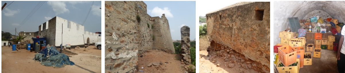
Figs. 88 to 91 – Encroachment (fig.88), cement plaster (fig.89), wall erosion (fig.90) and ancient dudgeons being used as storage (fig.91), can be observed in Fort Good Hope, in Senya Beraku.
