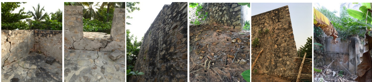
Figs. 214 to 219 – Structural problems are observed in the southern bastion (figs.214 to 216) and western bastion of Fort Groot Fredericksborg (fig.218). Termites are contributing to the soil settlement (fig.217). A shrine was built near the fort wall (fig.219).
