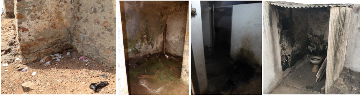
Fig. 53 to 56 – Fort exterior corners used as public toilet in Fort Good Hope (fig.53); interior space used as toilet in Fort Vernon (fig.54); existing toilets that are not working in Fort William (lighthouse) (fig.55); and open toilets in St. Jago in Elmina (fig.56).
