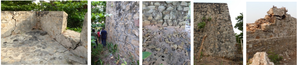
Figs. 16 to 19 – In Fort Groot Fredericksborg, the southeast bastion (figs.16-18) and the southwest bastion (fig.19) are sinking.
