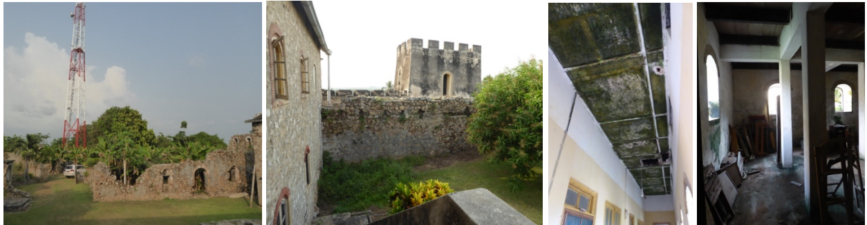
Figs. 210 to 213 – A high antenna lies at the entrance of Fort Groot Fredericksborg (fig.210); Humidity affects cement plaster (fig.211) and 2 nd floor ceiling (fig.212); concrete structure was introduced in several parts of the buildings (fig.213).
