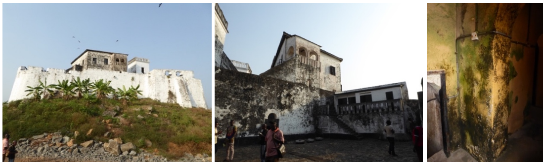
Figs. 220 to 222 – Lack of maintenance at Fort St. Anthony resulted in degradation of cement interventions and interior walls.
