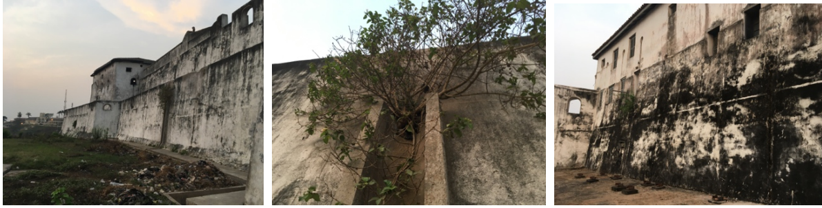
Figs. 47 to 49 – Neglect on clearing out gutters; and lack of wall cleaning and wall lime wash at St. Jago Fort walls
