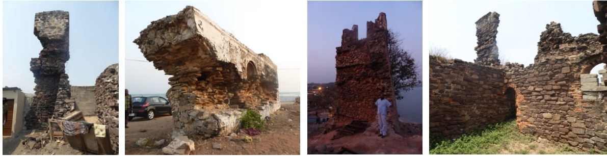
Figs. 1 to 4 – Structural instability of some of the walls in Fort Vredenburgh (Fig.1), Fort Fredensborg (Fig.2), Fort Nassau (Fig.3), and English Fort (Fig.4)
