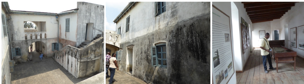
Figs. 227 to 229 – Lack of maintenance is observed in several walls (fig. 227 & 228); cement plaster intervention (fig. 228); and several interior exhibitions contribute for the community education and the fort interpretation (fig. 229), at Fort Apollonia.
