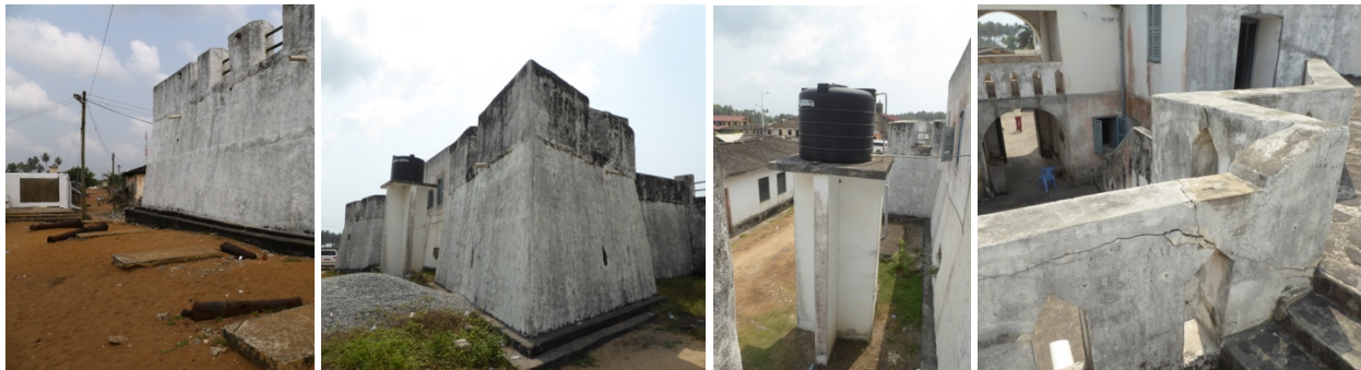
Figs. 223 to 226 – Abandoned cannons at For Apollonia (fig.223); Water storage jeopardises the fort's visual integrity (figs.224 & 225); structural instability of cement stair wall protection (fig.226).
