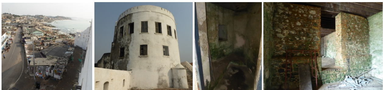
Figs. 127 to 130 – Encroachment near Cape Coast Castle (fig.127); occasional use of plastic paint instead of lime wash (fig.128); and interior rooms deterioration due to growing mould fungus originated from high moisture (figs.129 & 130). Historical dudgeons, where slaves were kept, should not be restored or limewashed. They should only be conserved, to avoid further deterioration.
