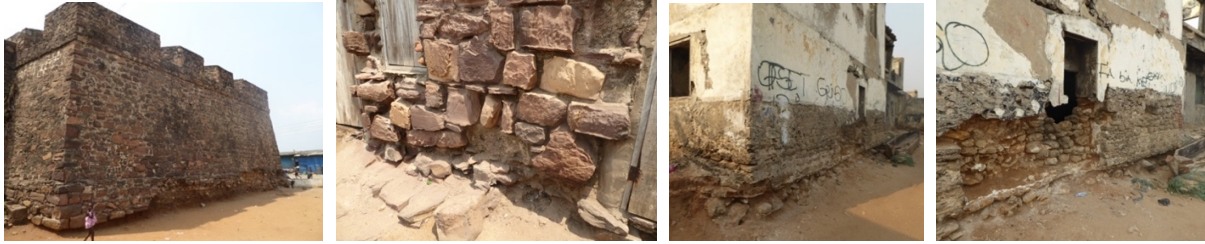
Figs. 21 & 22 – Sea erosion, removal of stones and exposed foundations are visible in English Fort (British Komenda). Figs. 23 & 24 – Erosion of the wall base and exposed foundations are also visible in Fort Vernon in Prampram.
