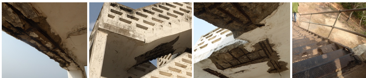
Figs. 135 to 138 – Concrete deterioration due to steel corrosion (figs.132 to 134). Corrosion of the metal stairs (fig.135).
