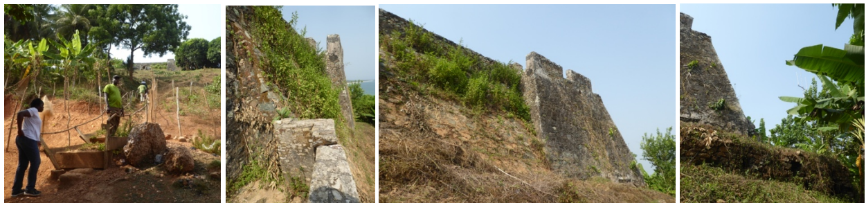
Figs. 187 to 190 – Access to Fort Batenstein is challenging and unstable (fig.187); the protective wall at the fort entrance is falling (fig.188); vegetation is growing in the fort walls (fig.189); and fort foundations are eroding in the south side (fig.190).
