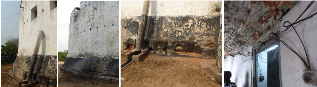
Figs. 139 to 142 – Problems resulting from water dropping at Fort William (Lighthouse) (figs.139 & 140); erosion on the basement of the exterior wall (fig.141); firebrick degradation on the basement vault and electrical unsecure wiring (fig.142).
