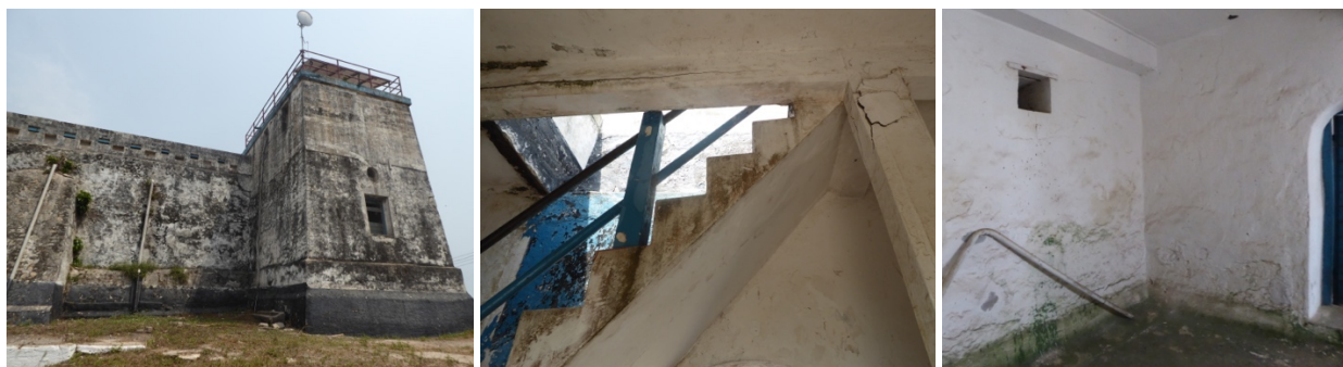
Figs. 184 to 186 – Fort Orange needs to have a better maintenance being regularly addressed (fig.184); especially as there are several problems with concrete beams in the interior of the fort (fig.185); there are new concrete ceiling interventions (fig.186).
