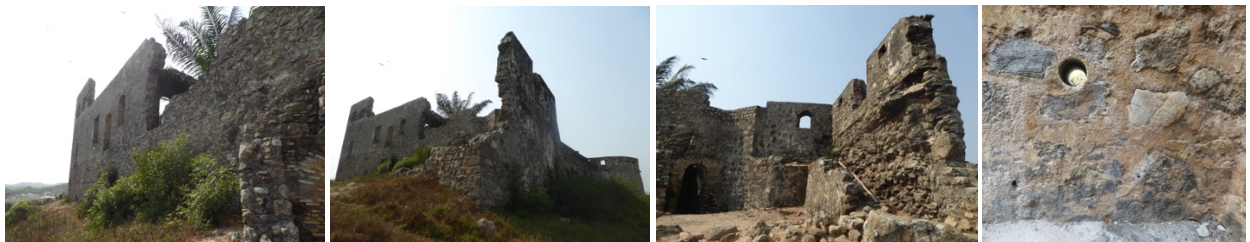
Figs. 101 to 104 – Need for structural consolidation in Fort Amsterdam (figs. 101 & 102), wall erosion (fig. 103) and a hole left by a drill when extracting soil for analysis (fig.104).
