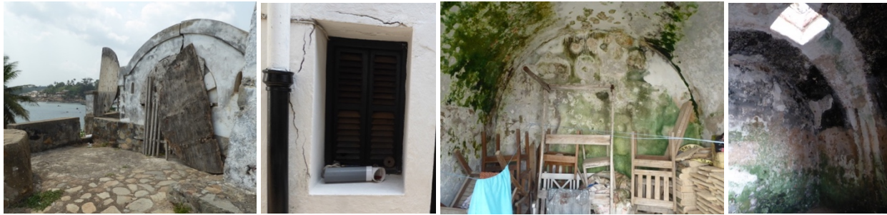
Figs. 198 to 201 – Structural problems at one of the entrances of Fort Metal Cross and at a new cement restoration (figs. 198 & 199); The slave dungeons are in bad state of conservation and are used nowadays as storage (figs. 200 & 201).
