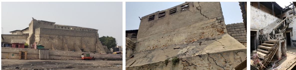
Figs. 85 to 87 – Fort James, in Jamestown is highly deteriorated, and damage can be already observed.
