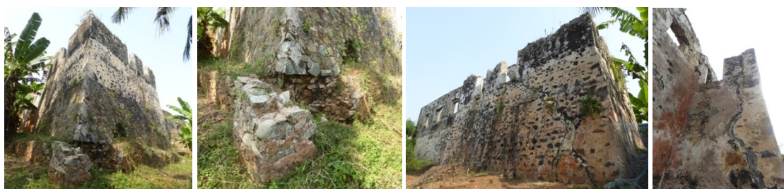
Figs. 191 to 194 – Several structural problems are potentially threatening Fort Batenstein stability.
