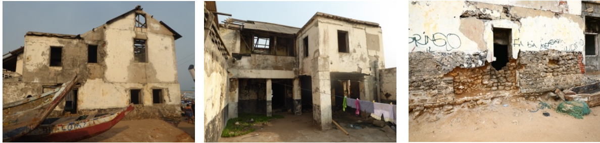
Figs. 70 to 72 – In Fort Vernon, cement additions from previous years, were followed by prominent neglect (figs.70 & 71). Decayed foundations of Fort Vernon (fig.72).
