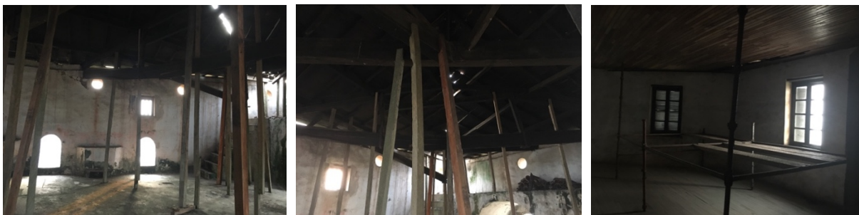
Figs.9 to 11 – The roof wooden structure is falling in the northwest and the ceiling in the northeast of Fort St. Jago, in Elmina.
