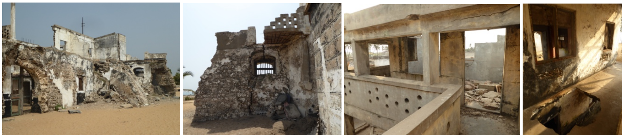
Figs. 5 to 8 – Structural instability in Fort Prinzenstein (Figs.5 & 6) and Fort Vernon (figs.7 & 8)
