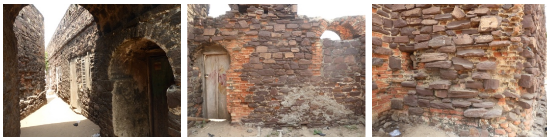
Figs. 166 to 168 – Some parts of Fort English are standing and are still in good condition (fig.166); however, other parts are facing high erosion especially regarding the exposed mortar from the stone masonry (figs. 167 & 168).
