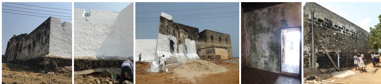
Figs. 92 to 96 – Lime wash at Fort Patience is hiding fungus on the walls and structural issues that need to be addressed.
