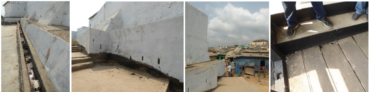
Figs. 173 to 176 – At Fort St. Sebastian gutters need to be cleaned (fig.173); some fort foundations are exposed (fig.174); there is some encroachment (fig. 175), and there is some wooden unstable pavement in the second floor of the fort (fig.176).
