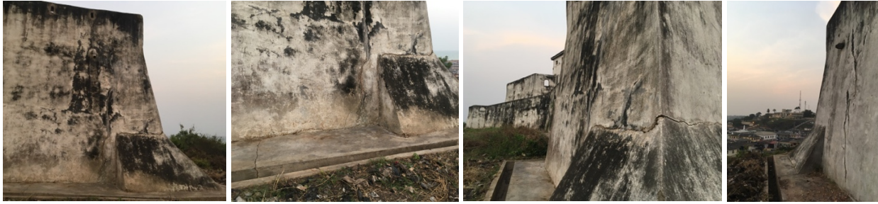
Figs. 12 to 15 – In St. Jago Fort, the northwest bastion is sinking due to unstable ground.
