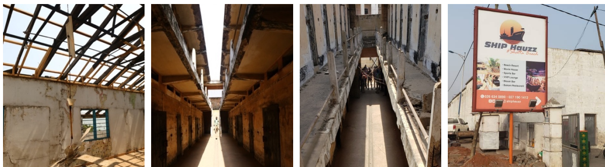
Figs. 81 to 84 – Ussher Fort, in Usshertown is highly deteriorated and needs urgent intervention (figs.81 to 83). A wide signpost, at the entrance of the fort, doing publicity to a Beach Resort, also interferes with the site interpretation (fig.84).
