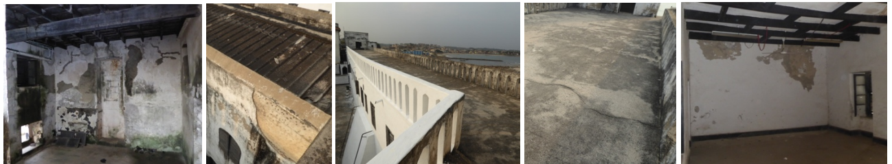
Figs. 152 to 156 – In St. George Castle in Elmina, lack of maintenance resulted in interior degradation (fig. 152); wall degradation (fig.153); terrace structural instability (figs.154 & 155), which caused unstable beams underneath the roof terrace (fig.156).
