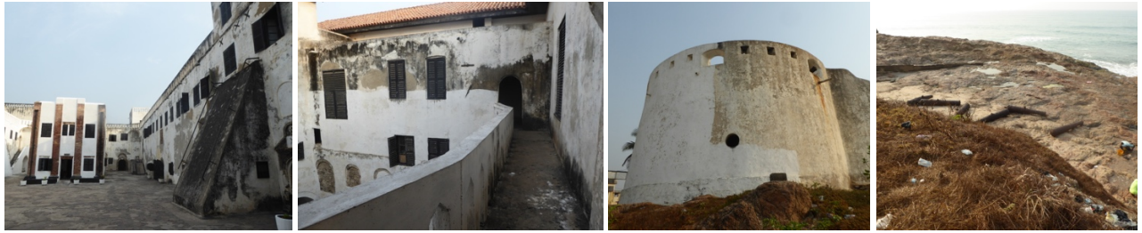
Figs. 148 to 151 – In St. George in Elmina, lack of maintenance is observed (fig.148), in spite of the partial lime-wash, which has not been concluded (figs.149 & 150). Cannons are also abandoned in the beach, in the surroundings of the castle (fig.151).
